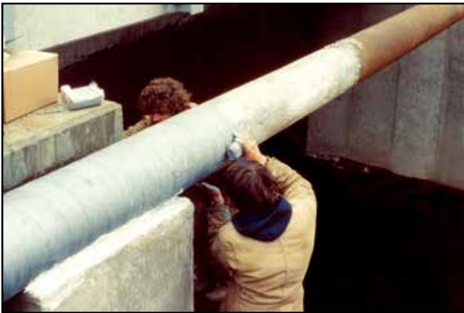
Here Trenton's Wax-Tape® #2 wrap is being applied over the Wax-Tape® primer (white). Notice that the Wax-Tape primer can be applied to the pipe after only minimal surface preparation.
